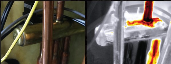
FAILING REVERSING VALVE
