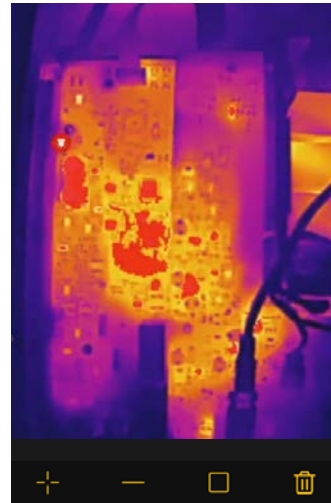
Over-temperature area alarm
